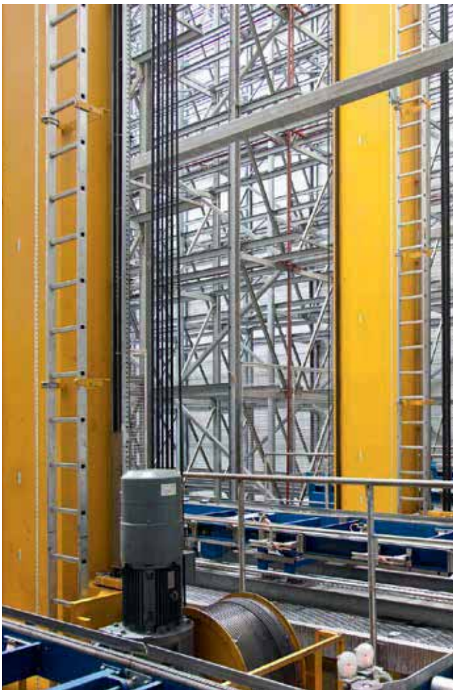
Storage/retrieval system (SRS)
